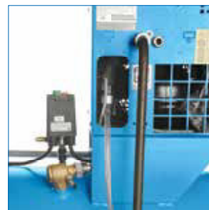
Pre-installed and connected
